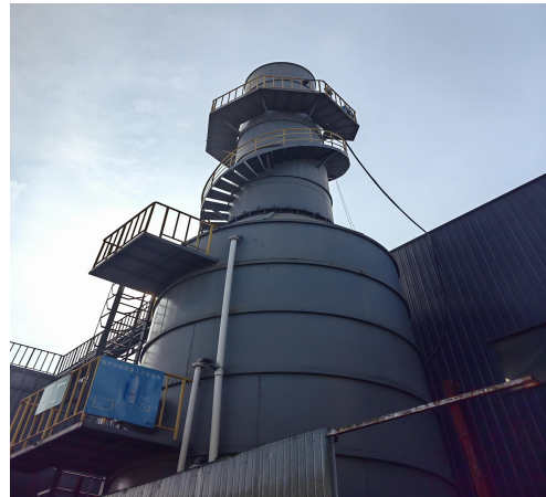
碱喷淋塔、DA001 排气筒
